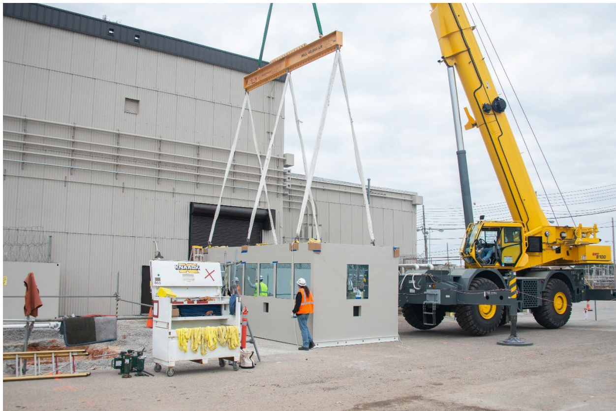
The recently delivered Security Inspector's Operation Area, seen here being moved into the main production area in K Area, will allow remote inspections of employees working on the upcoming Surplus Plutonium Disposition mission.
