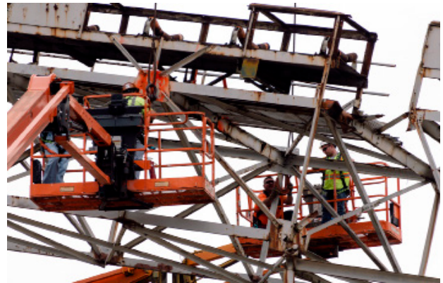
A team with Savannah River Nuclear Solutions mentor-protégé company CTI Associates works to dismantle a decades-old structure at the Savannah River Site for recycling.
