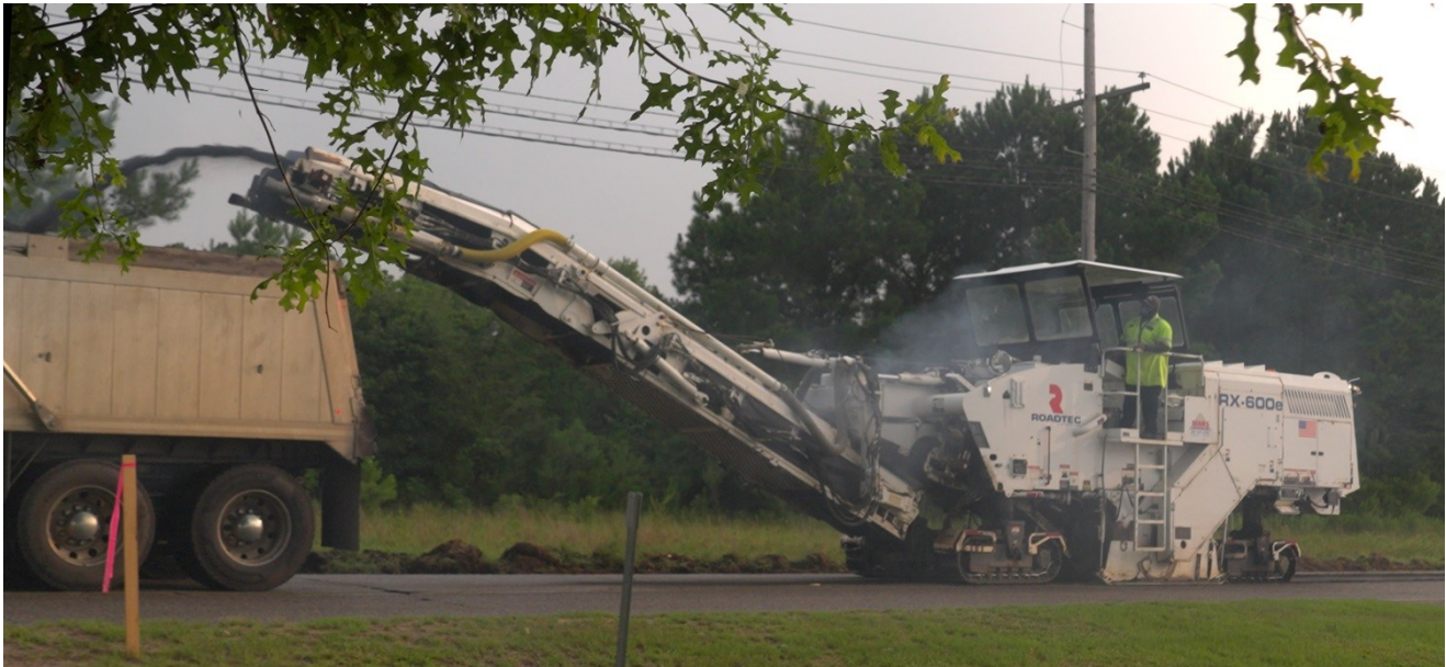
A milling machine at the Savannah River Site (SRS) removes cracked and aged asphalt to ensure a strong foundation for the new road surface.
