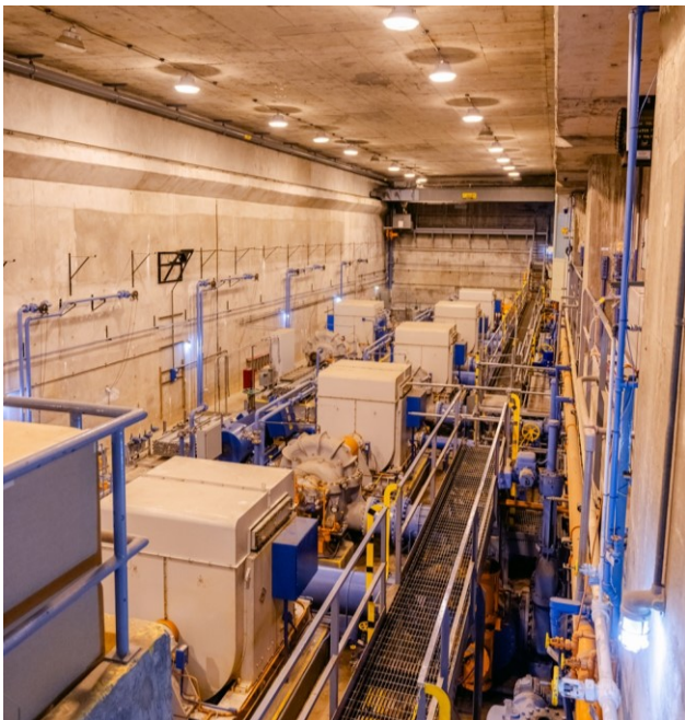
Managing water infiltration in the underground valve pits helps maintain the D Area River Water Pump House, which provides surface water across the Savannah River Site.
