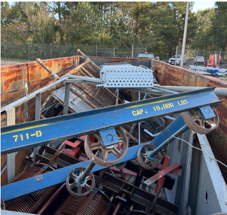
Over 47,000 pounds of scrap metal were recently recycled as part of a switchgear replacement project at the Site’s River Water Pumphouse.
