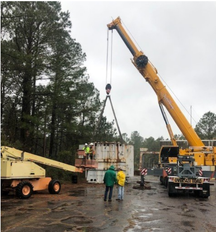
SRNS excessed five transformers and donated them to the Savannah River Site Community Reuse Organization.
