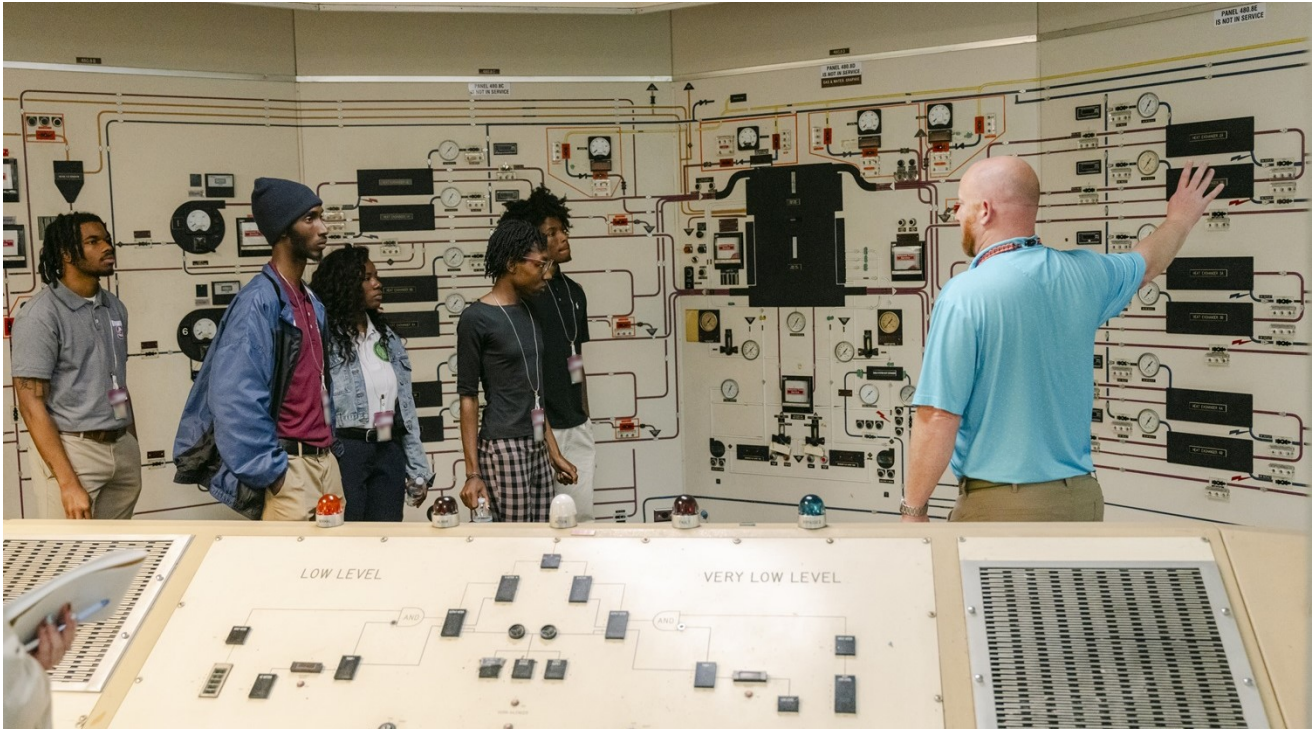
South Carolina State University students were particularly interested in the legacy control panels found in L Area.
