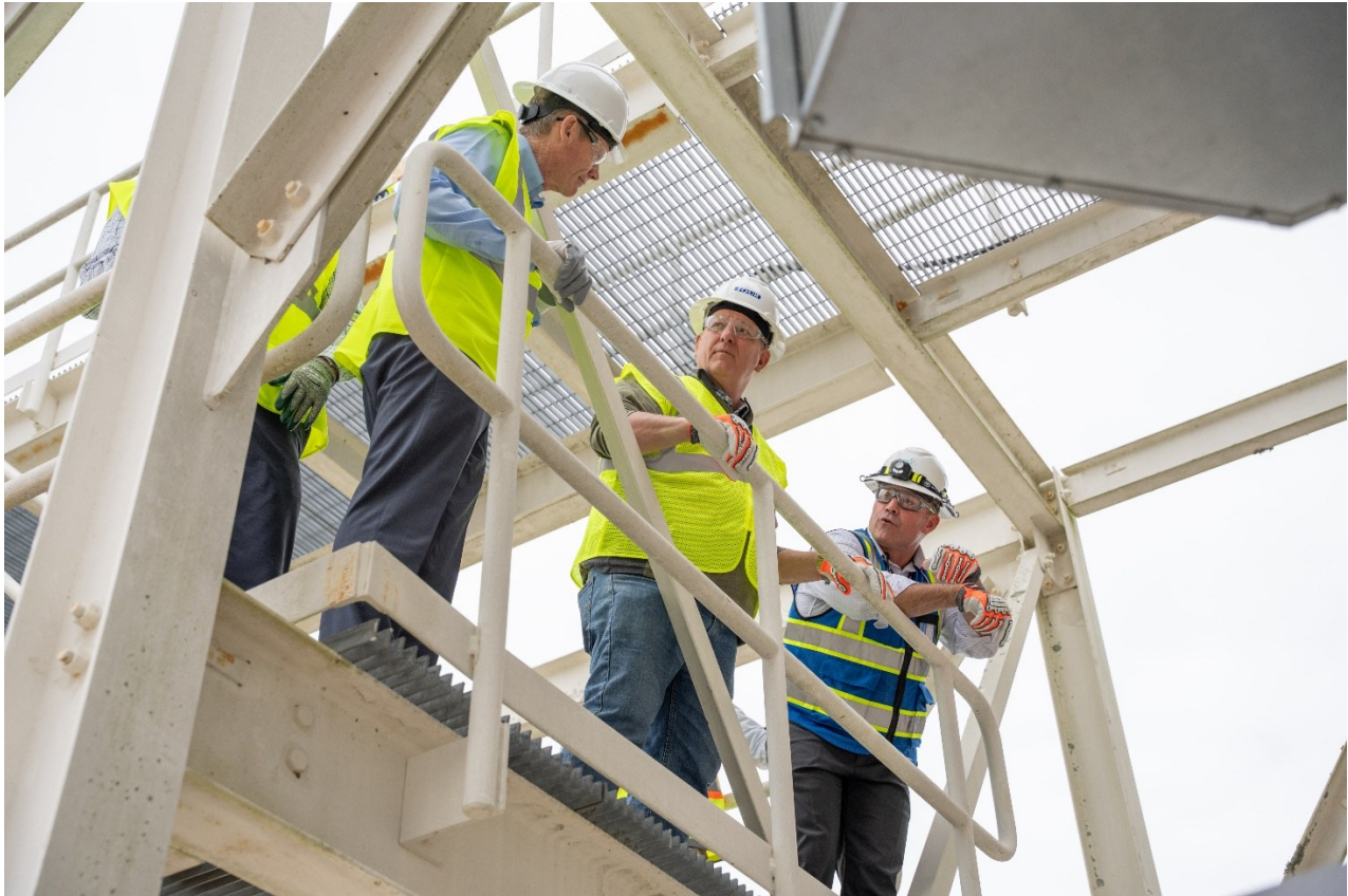
NNSA Principal Deputy Administrator Scott Pappano, center, stands atop the Savannah River Plutonium Processing Facility (SRPPF) while viewing site preparation progress with SRNS Executive Vice President and Chief Operations Officer Jim Dawkins, left, and SRNS Senior Vice President of SRPPF Project Execution and SRPPF Project Director Mike Basham.
