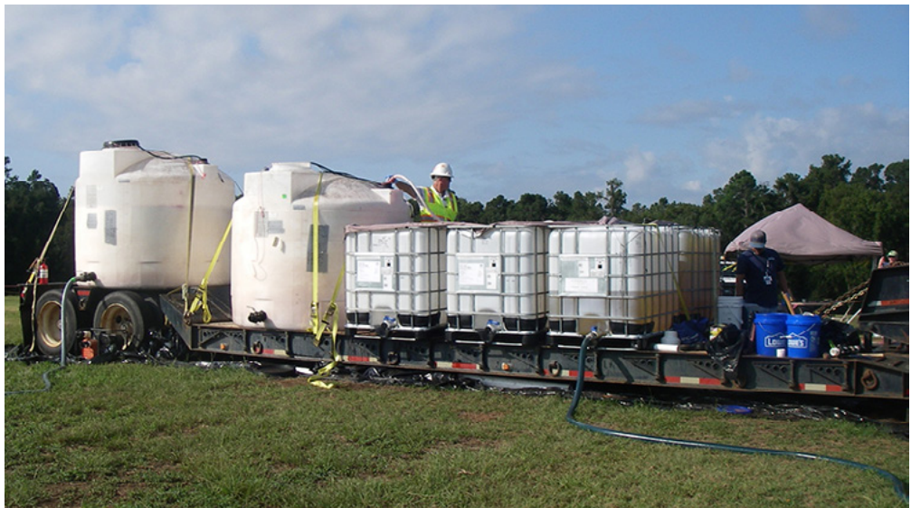
North Wind, a small business contractor for Savannah River Nuclear Solutions (SRNS), treats groundwater at the Savannah River Site in Aiken S.C. SRNS has surpassed its small business contracting goals for fiscal year 2016, awarding more than $177 million to small businesses.
