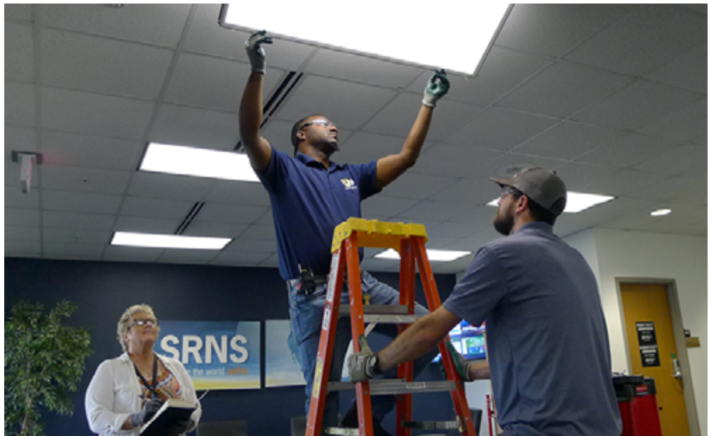
Savannah River Nuclear Solutions (SRNS) Facility Manager Cheryl Parrow monitors the relamping of an SRS administrative facility by SRNS mentor-protégé company US&S, Josh Miller (center) and Matthew Bradham inspect a new fixture.
