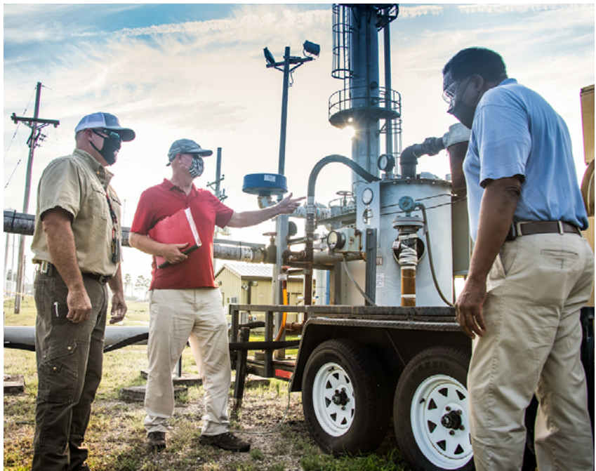
Savannah River Nuclear Solutions mechanic Todd Cockrell, Engineer John Bradley and Project Manager Joao Cardoso-Neto plan the removal and dismantlement of a high-vacuum soil vapor extraction unit at the Savannah River Site’s M Area.
