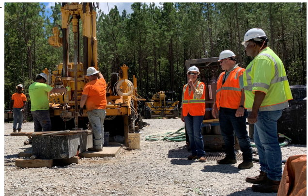
Using an innovative metal piercing device and cement-like grout, Savannah River Nuclear Solutions (SRNS) saved about $900,000 in a project that safely closed a 70-year-old well at the Savannah River Site. Karen Adams, third from right, DOE-Savannah River federal project director, discusses progress on the project with Allen Henderson, far right, SRNS subcontract technical representative and Joao Cardoso-Neto, SRNS project manager, Area Completion Projects
