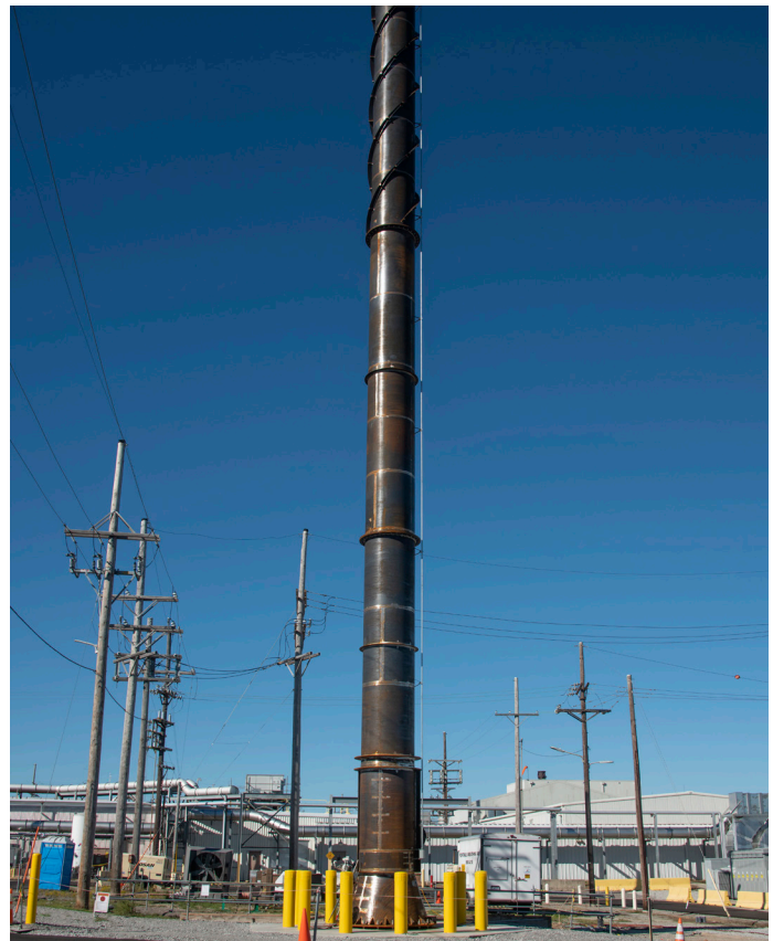
New exhaust stack erected as part of the multiphase project to provide new exhaust ventilation for the Savannah River Tritium Enterprise’s Materials Testing Facility lab
